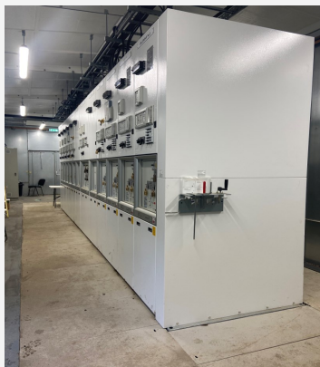
SPEN Primary Sub Switch Room
